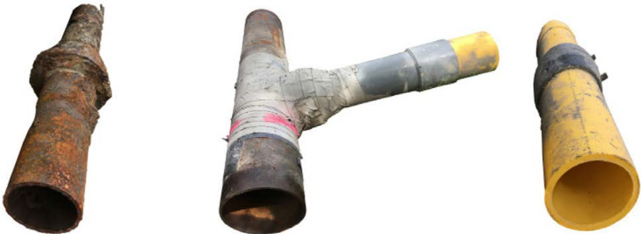
Figure 1. Examples of pipe materials recovered from underground. From left: cast iron, bare steel, and plastic.
